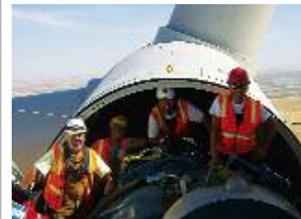
Working "on top of the world" at Local 112 wind turbines project outside Athena, OR, are, from left: Jerry Fletcher and Arnie Langendoerfer, Local 280; "Pistol" Pete Nevin, Local 332; and Tim Hittner, Local 280.
